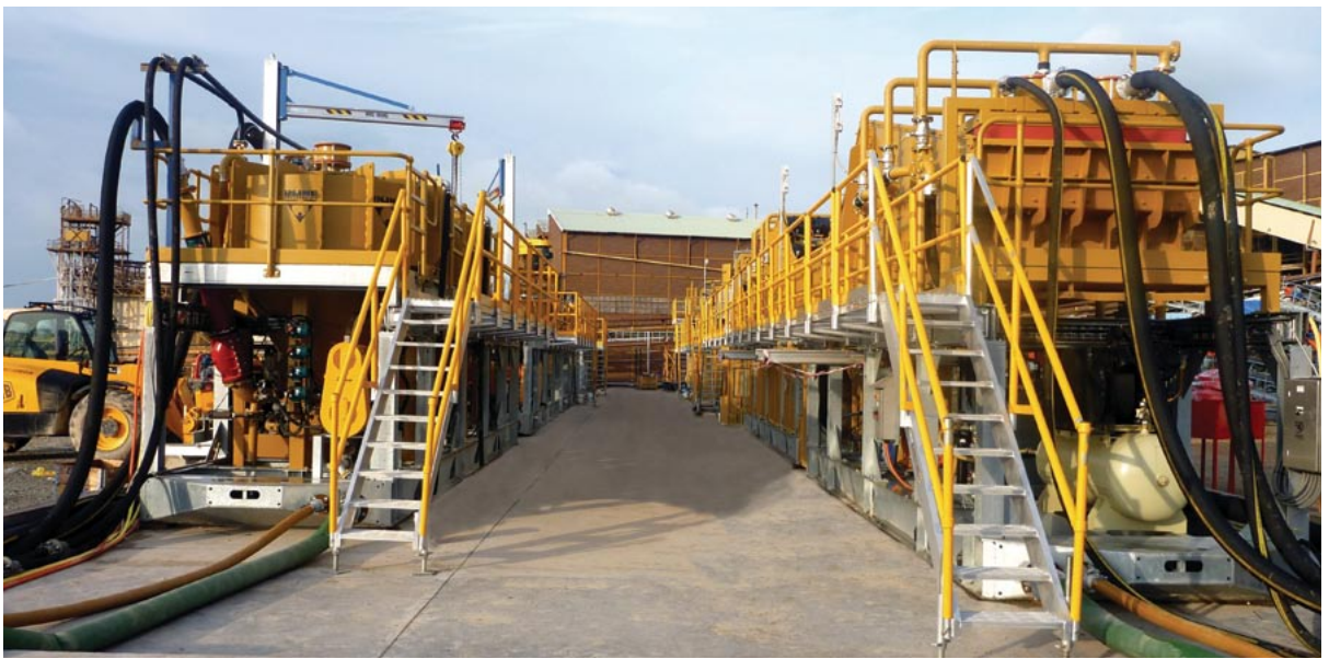
The Python 500 modular plant installed at the Gold Fields Kloof GROWTH Project
