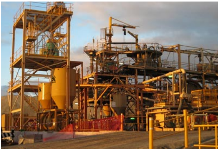
Gold Fields' Agnew project - an example of Gekko's ability to provide a turnkey solution
